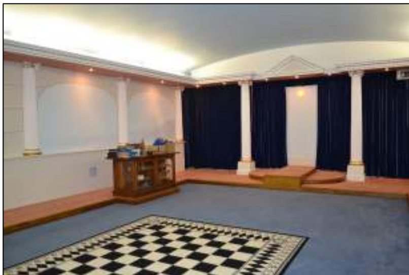
Pictures taken during the redecoration as a result of water damage in the St Martins Lodge Room
